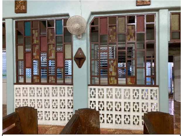
To help with ventilation, the walls are designed to let air flow through from the open porch outside. The electric fans are still much appreciated!
